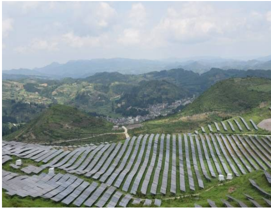
A photovoltaic power station (solar farm) in Emaozhai Village, Baotian Town, Panzhou City, Guizhou Province, China Source: Xinhua News Agency
